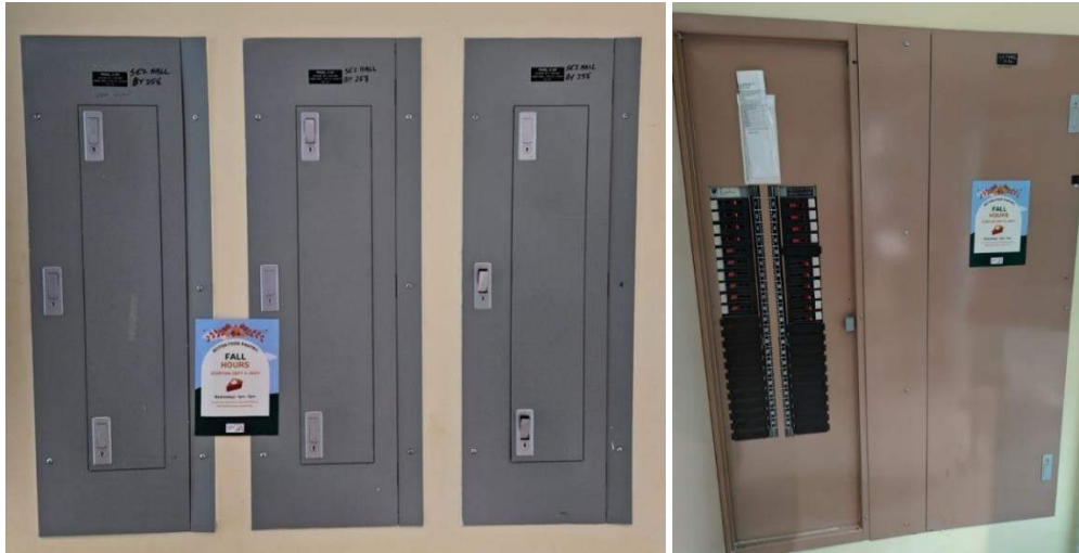
Figure 8: Existing Panels 2-2H, 2-2C, 2-2B, 2-4A and LV Relay Panel 2-4A on Level 2
