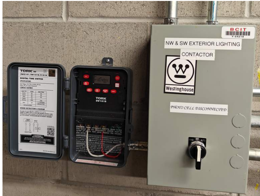
Figure 10: Existing Timeclock at the Main Electrical Room
