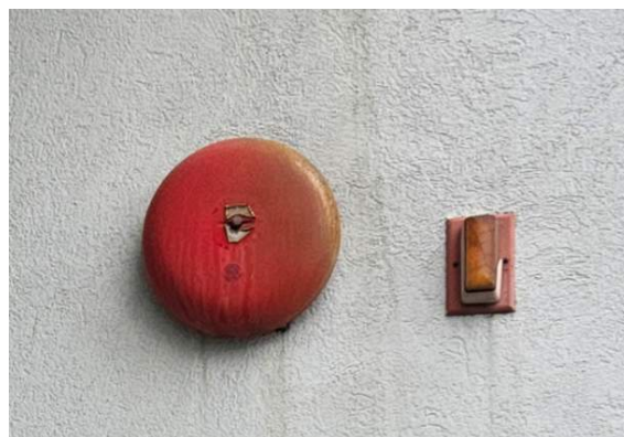
Figure 17: Existing Fire Alarm Gong and Strobe at the Patio Space
