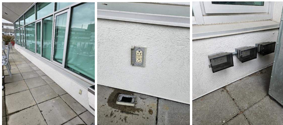
Figure 13: Exterior Receptacles at the Existing Patio Chamber
