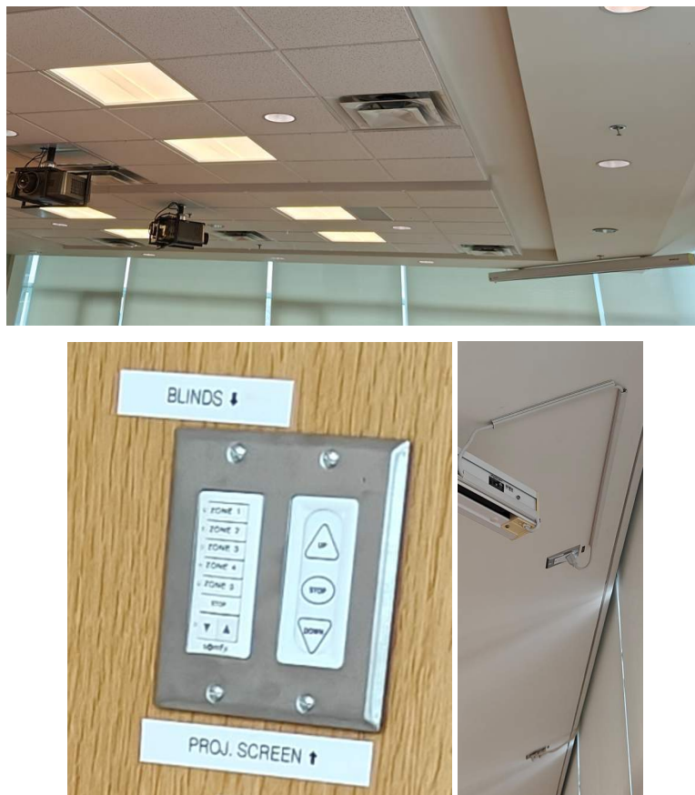
Figure 15: Existing Projector Screen, Motorized Blinds and Receptacle Connections
