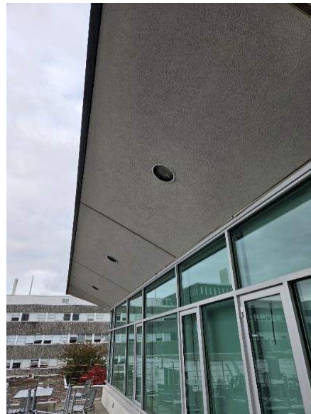
Figure 9: Existing Exterior Downlights at the Canopy
